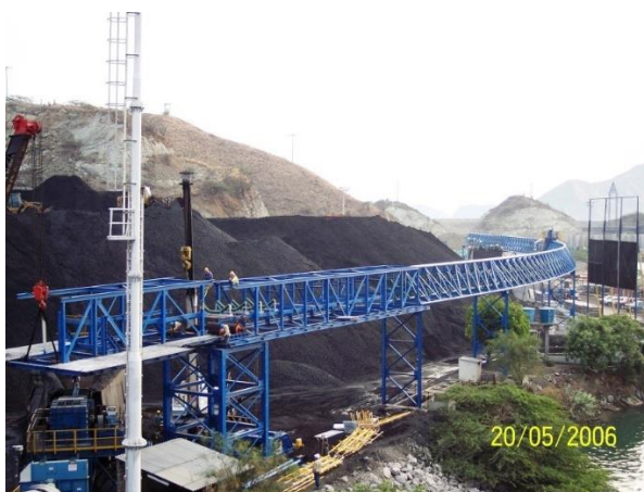
Figure 14. Pipe Conveyor with Triangular Frame and Maintenance Trolley
