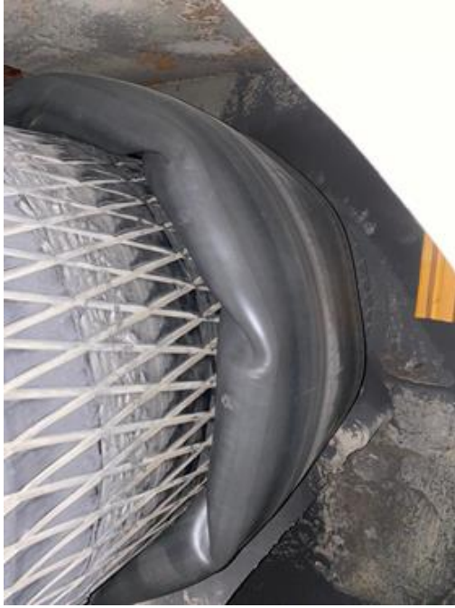
Figure 12. Belt folded over the head pulley of a pipe conveyor
