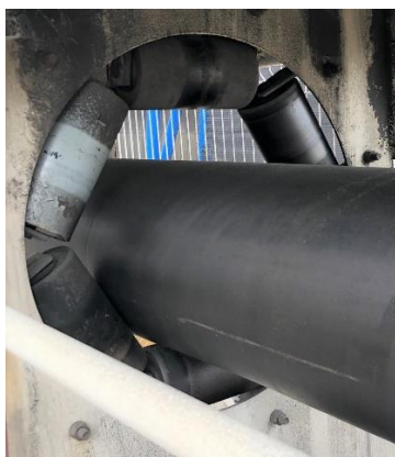
Figure 4. “Normal” belt recently installed in a Pipe Conveyor
