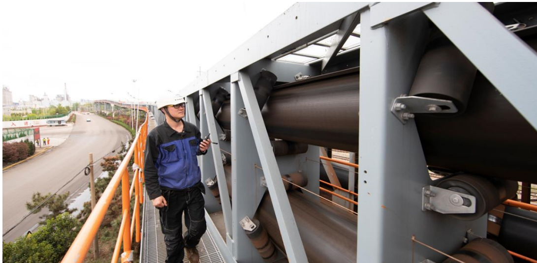
Figure 2. 5,500 tph Pipe Conveyor for Iron Ore
