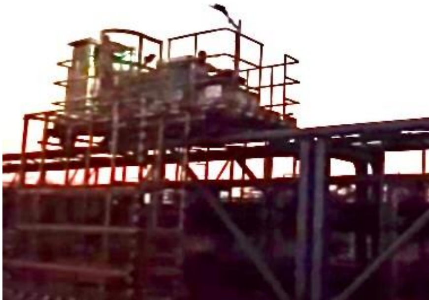
Figure 15. Pipe Conveyor with Rectangular Frame and Maintenance Trolley
