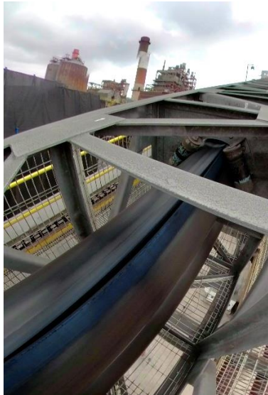
Figure 5. “Pipe” belt recently installed opening between panels due to excessive stiffness.
