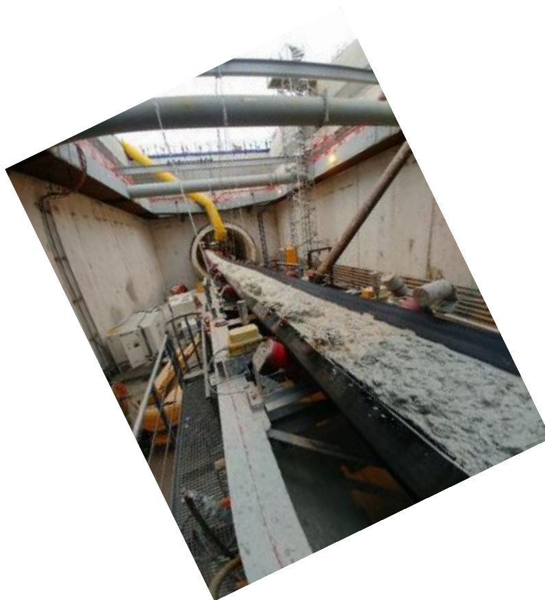
Figure 9 – Conventional TBM trailing conveyor at the Paris Metro project.
