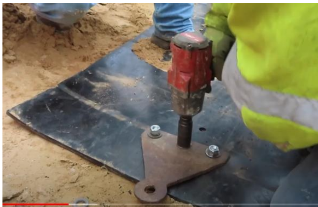
Figure 16 - Cleat bolted to belting - not certified
