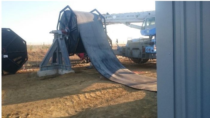
Figure 10 - Belt unreeling facility
