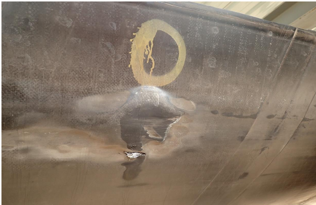
Figure 7, Project example 1 "Bubble" in the splice due to cord pull-out
