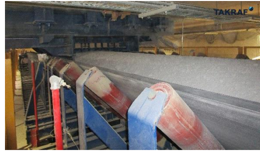
Figure 3: Feeder conveyor – picture.
