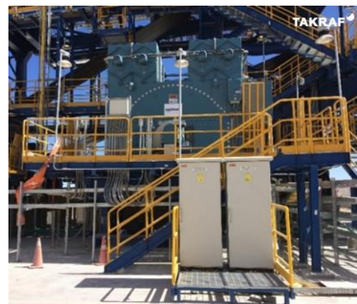
Figure 7: 5 MW drive as installed.
