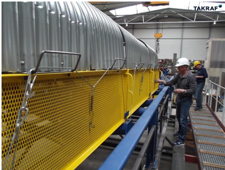
Figure 21: Belt cover sample installation at the workshop and fabrication facility in Lauchhammer, Germany.
