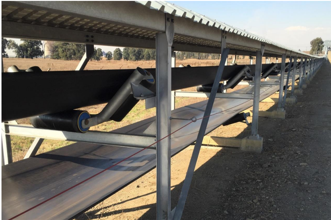
Figure 7. Idler and stringer arrangement along the conveyor.
