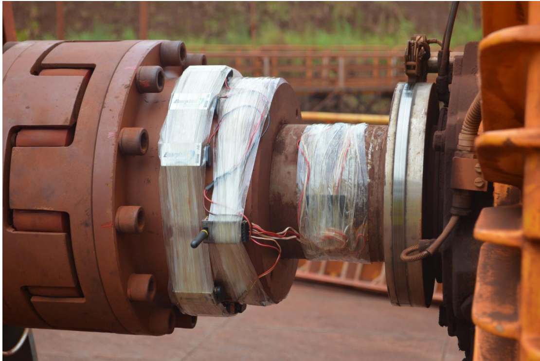
Figure 20. One of the 24 shaft torque measurements installed during commissioning.
