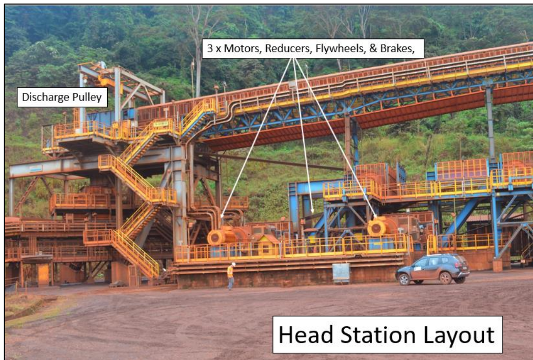
Figure 14. Head drive layout for conveyor TR-2011KS-07.
