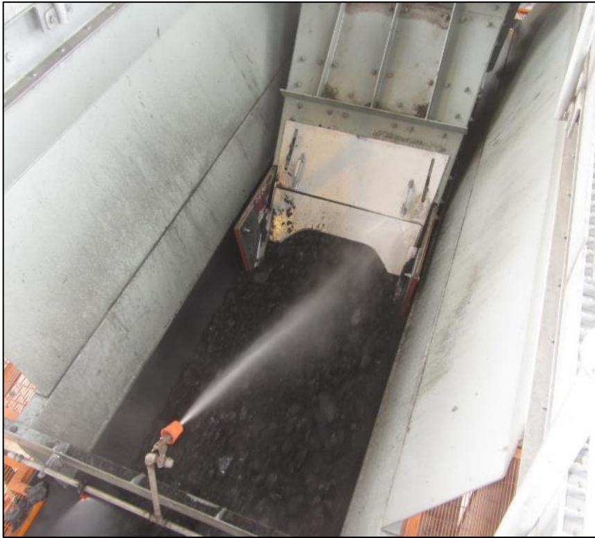
Figure 9: Lowered luffing chute feeding coal onto the reclaim conveyor
