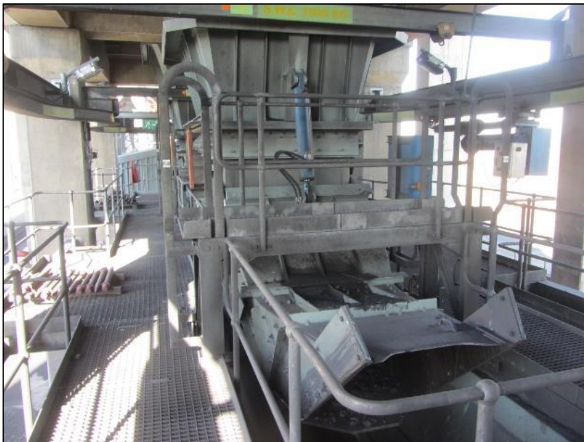
Figure 8: Luffing chutes underneath the bunker
