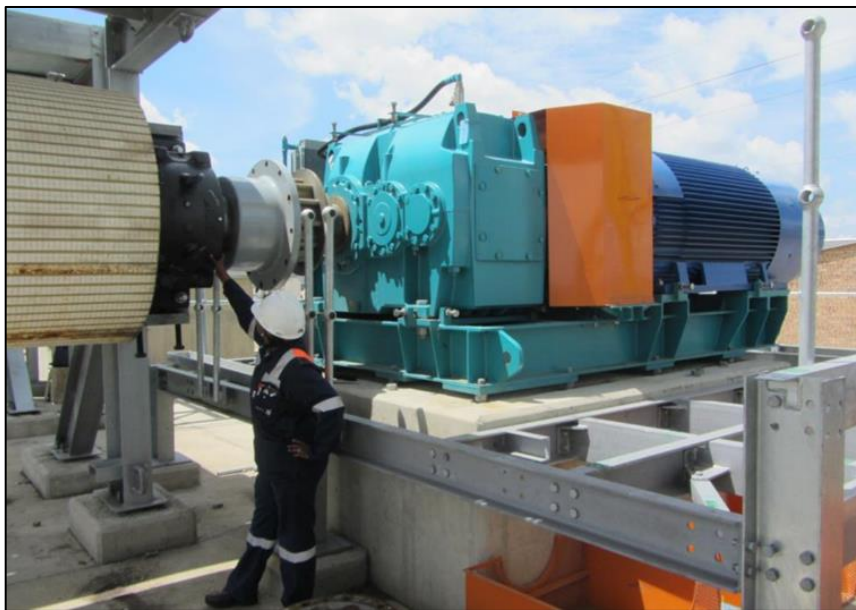
Figure 4: Impumelelo overland conveyor intermediate drive
