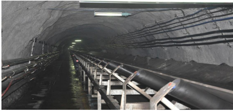
Figure 7. Aramid DPP 2000 belt in Baodian Coal Mine (YCMC), China.
