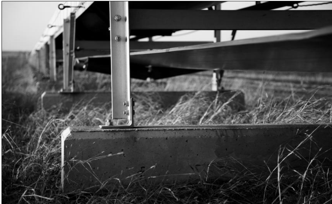
Figure 5. Overland concrete sleepers
