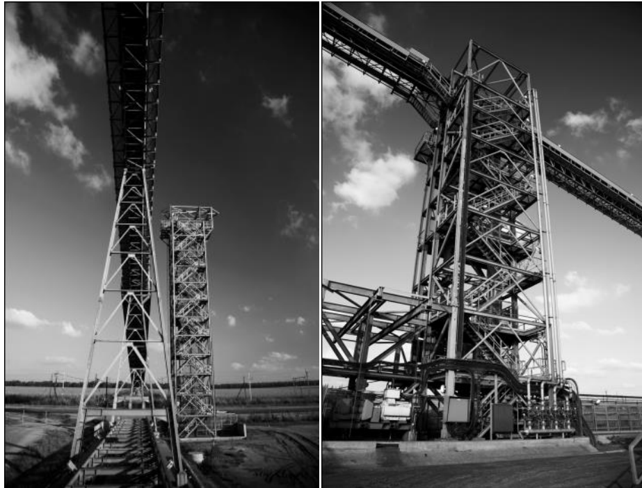
Figure 3. Take-up tower and vertical belt turnover
