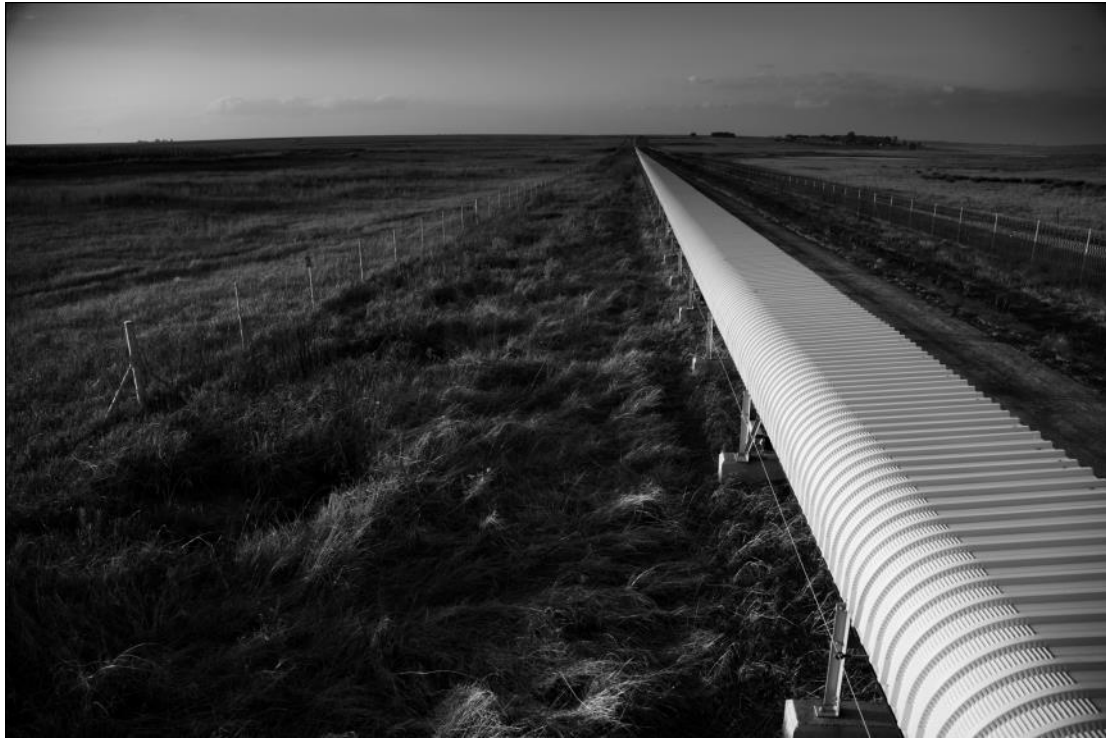
Figure 2. CV0004 with doghouse sheeting
